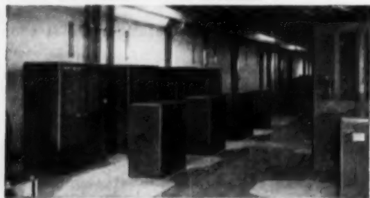
Pickling Line V*S Drive Control Units
